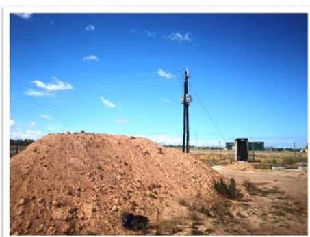
Eskom electricity connection
